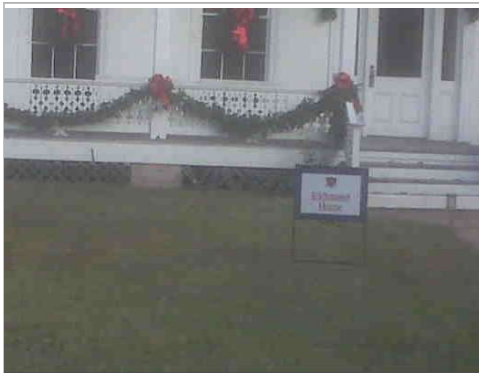
Repair/replace/paint broken green lattice
