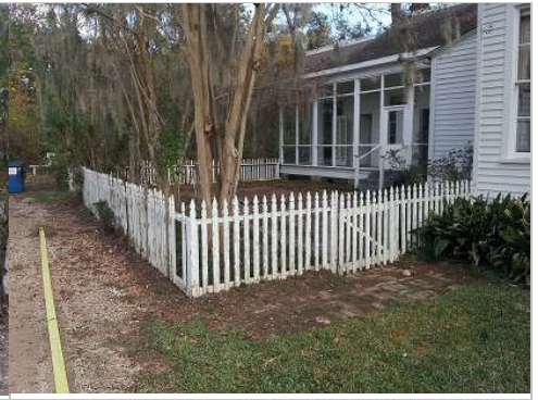
Repair/Replace broken & rotted fence posts & paint fence
