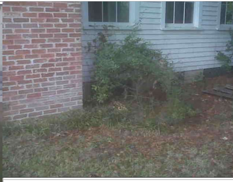
Remove brush & repair/paint green lattice
